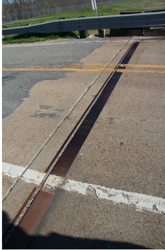
Condition Photo 10: Concrete deck expansion joint at north abutment.
