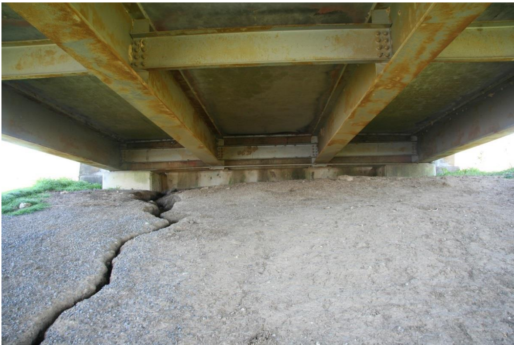
Condition Photo 7: Erosion under northerly most approach span at north abutment; also shows condition of failed paint system on structural steel members.
