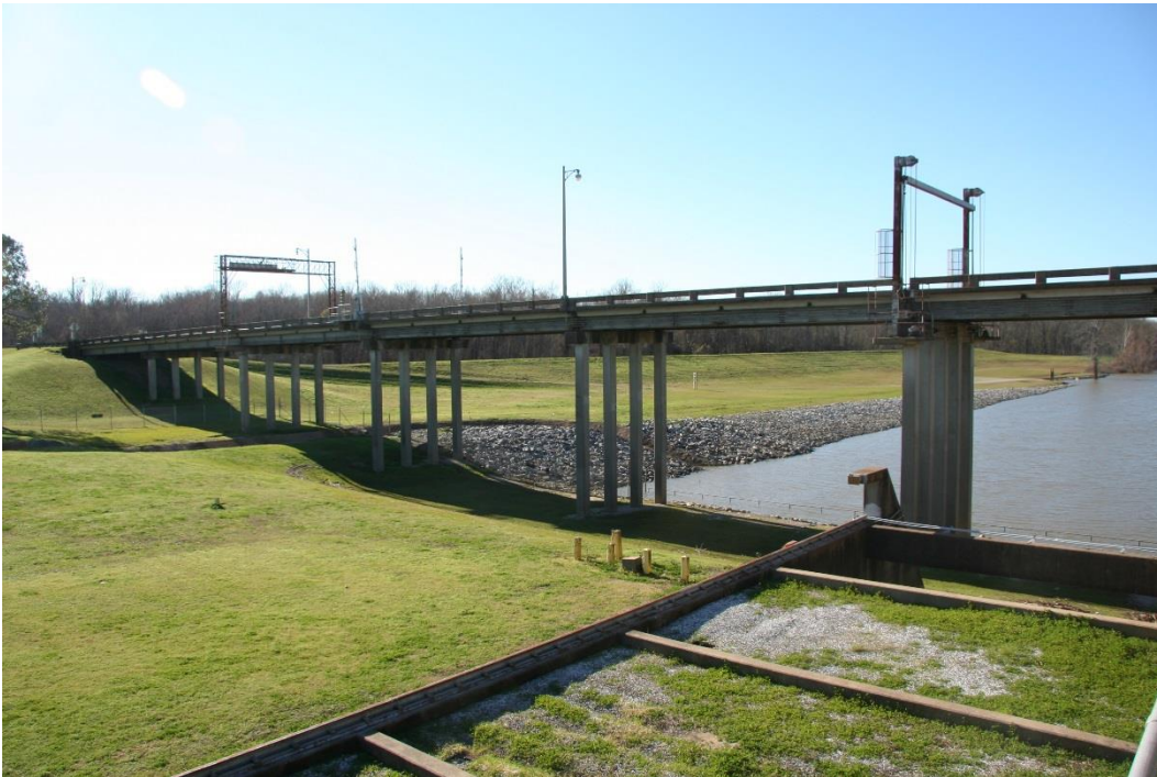
Historic Fabric Photo 1: Typical steel plate girder approach spans with concrete railing and concrete pile supports, showing traffic gates.
