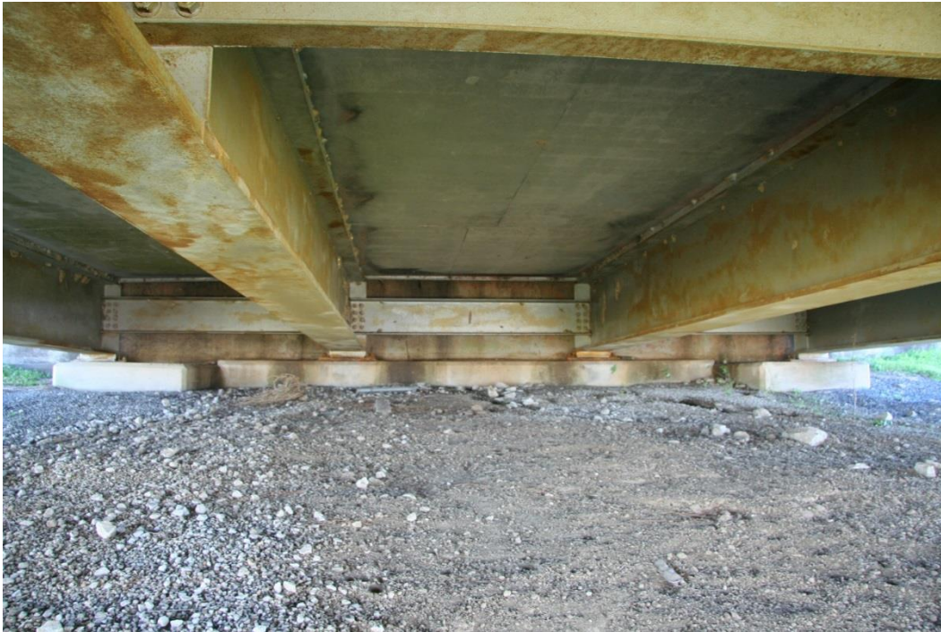
Condition Photo 18: Underside of south approach spans at south abutment; also shows condition of failed paint system on structural steel members.
