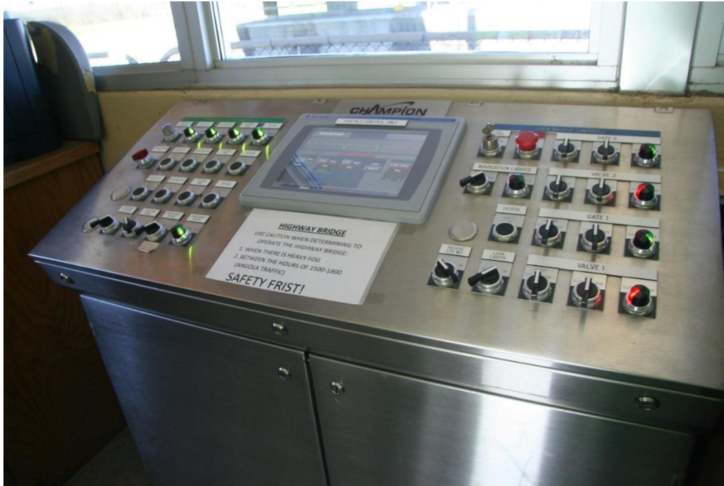
Photo 20: Control panel, PLC controls.
