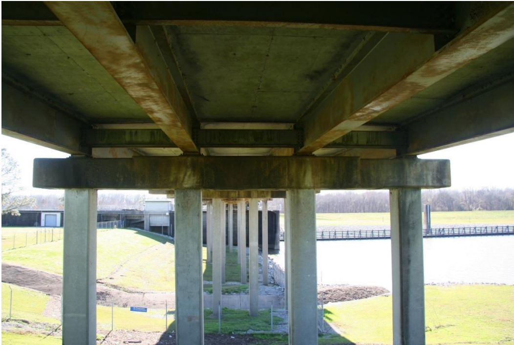
Condition Photo 6: Underside of north approach spans, looking at Bent 10; also shows condition of failed paint system on structural steel members.
