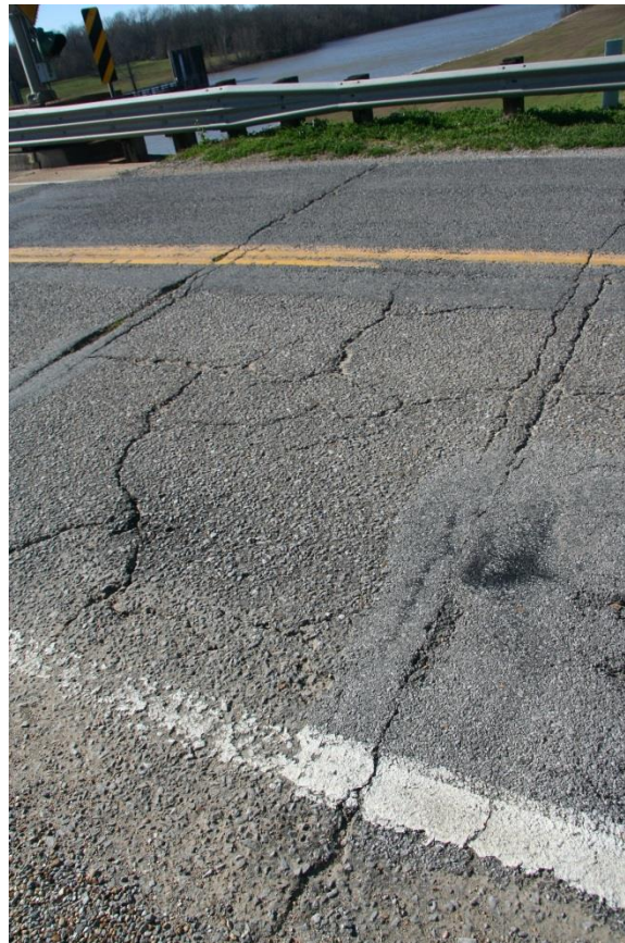
Condition Photo 5: Condition of road at north approach to bridge.
